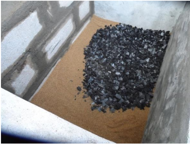
Picture 4: Set-up of the bottom layer and the intermediate layer of the drainage layer, i.e. 15 cm of sand and 5 cm of charcoal, Liberia.
