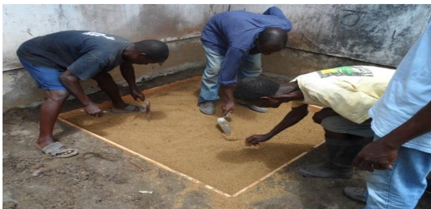
Picture 1: Building of a concrete foundation for an above ground biodigester, Liberia.
